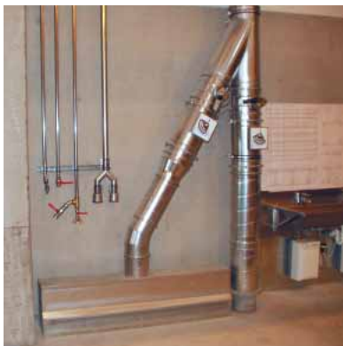
Dust extraction with an application specific pipe system
