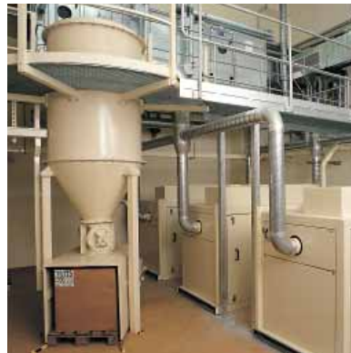
Filter system with dust removal through rotary valves and parallel operating rotary piston blowers
