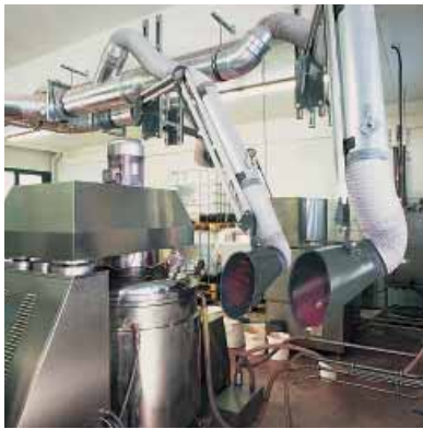
Source capture with two extraction arms
