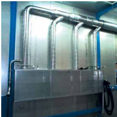
Extraction hood inside a sanding cabinet
