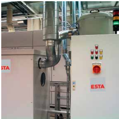
Control unit with monitoring lamps
