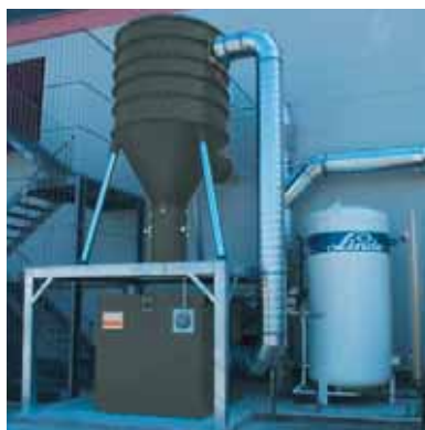
Two cyclonic filters as part of an extraction system
