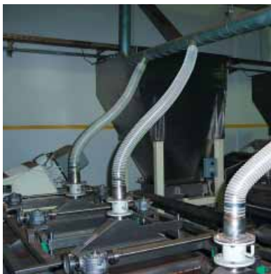
Capturing of the dust above the conveyor belts
