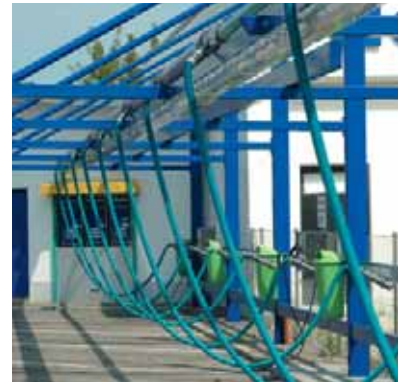
A rigid pipe installation connects the vacuum locations with the cyclonic filter
