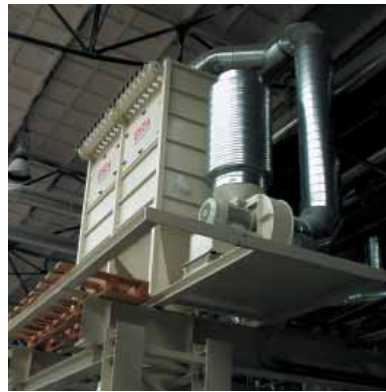
Tubular bag filter unit with separate extraction fan unit
