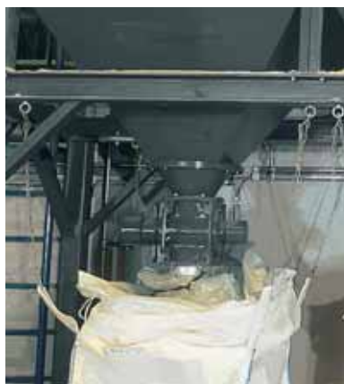
Removal through rotary valve
