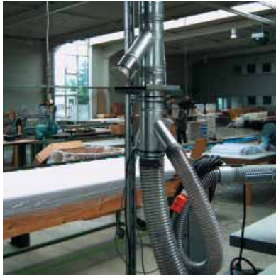
Pipe system with connection for extraction hoses
