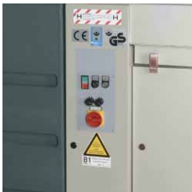
Clearly laid out control panel for easy operation.
