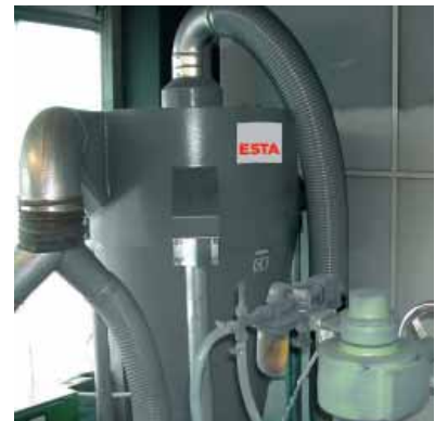
Cyclone ZA 160 in operation
