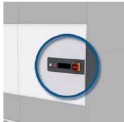
Clearly laid out operating console
