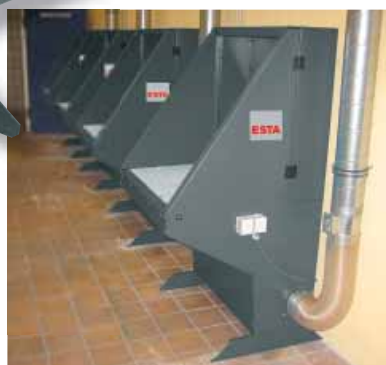
Multiple ESTA welding tables connected to an extraction and filtration system
